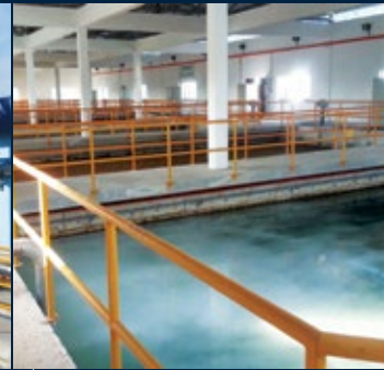
Dissolved Air Flotation (DAF) Tanks
