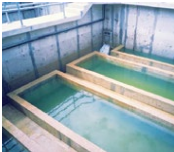
Lamella Plate Clarifiers
