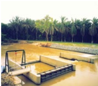
Rubber Weir across Sg. Muar
