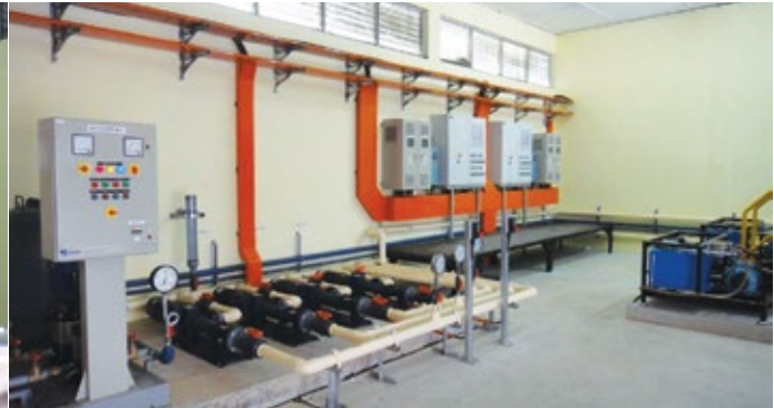
Switch Board & Polymer Transfer Pumps in Sludge Decanter Building
