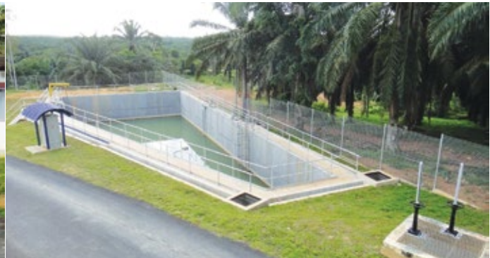
Sludge Holding Tank
