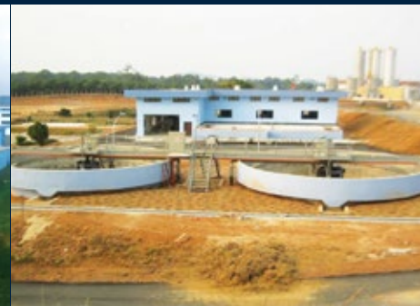
View of Wash Water Recovery Tank & Pumping Station and Sludge Thickeners
