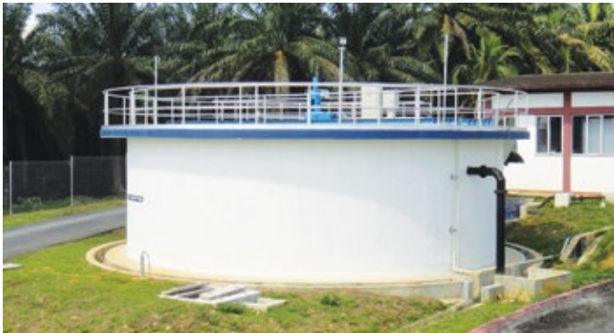
Sludge Thickener Tank
