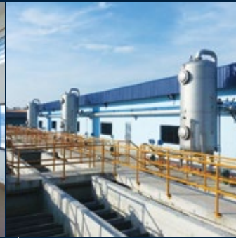
View of Flocculation Tanks and Dissolved Air Flotation (DAF) Building
