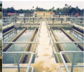
Overview of Aerator, Flocculation Tanks and Clarifiers
